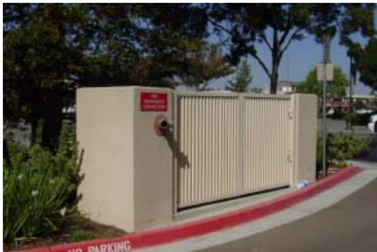
Backflow preventor is screened by wall and landscaping.
