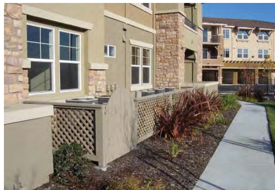
Air conditioner units screened behind landscaping and screen walls
